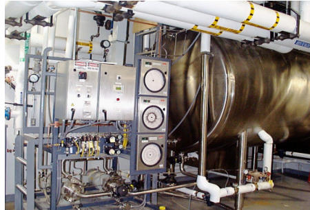
WFI Tank and Pump Skid
