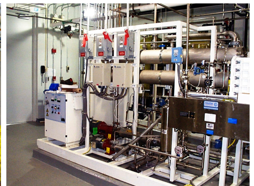
Reverse Osmosis System
